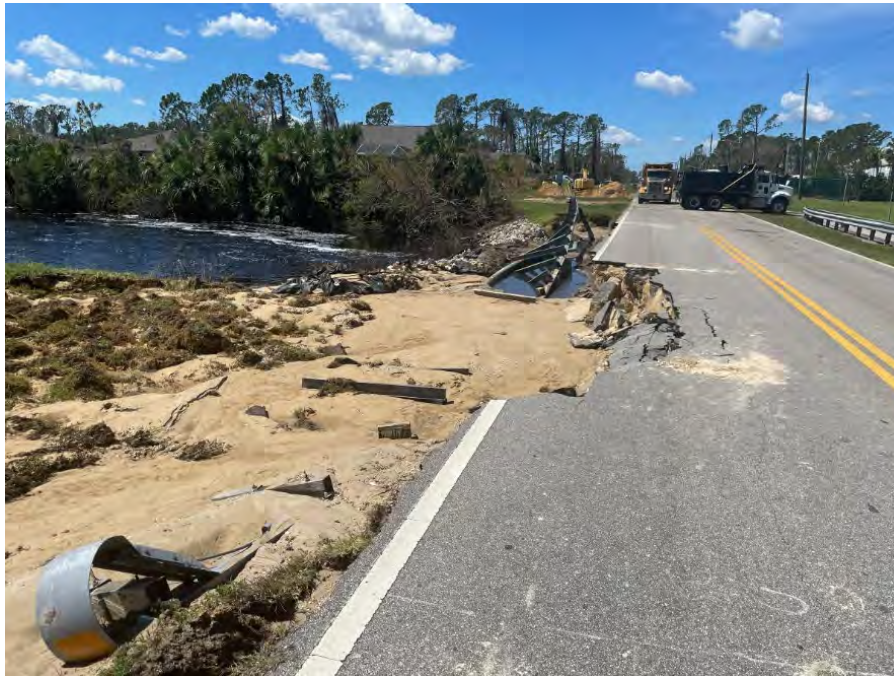
Figure 17: Roadway damage and partial washout near the Myakka River in North Port, Florida 88
