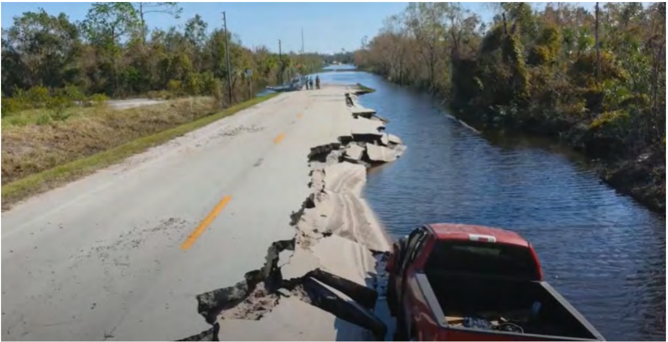
Figure 19: Significant roadway damage in DeSoto County along the Peace River 90
