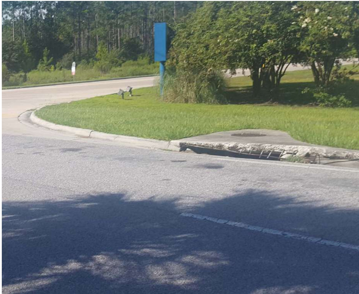
An example of the extensive curb damage that can be seen throughout the County and City as trucks navigate through narrow streets to the Interstate.
