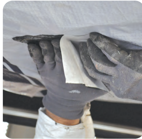
6. Apply waterproof, permanent adhesive to patch for belly wrap, with patch sized at least 3 inches larger than hole in barrier
