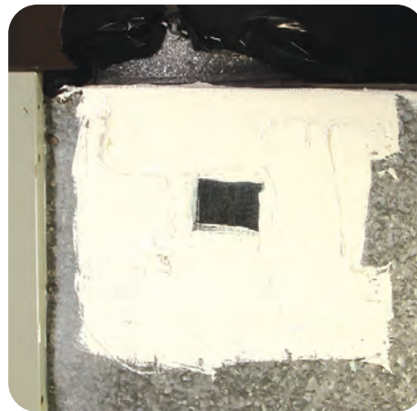
C-4. Apply additional mastic over mesh, extending at least 1 inch past tape and seam in all directions
