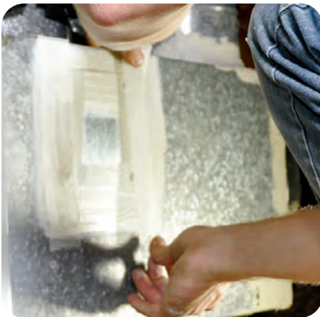
C-3. Apply mastic over edges and fasteners of patch and push fiberglass mesh into it
