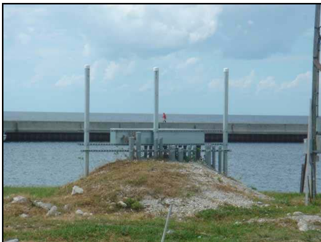
Figure 1 shows elevated utilities at the Everglades Adventures R.V and Sailing Resort. Simple and Inexpensive techniques, such as this, can mitigate flood impacts. Source: CSA, 2006
