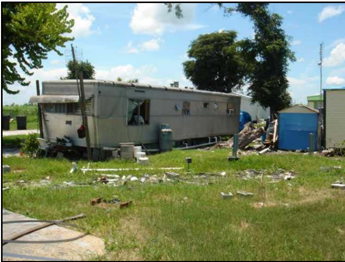
Figure 3 shows an substandard farm worker rental residence in the Glades Communities. This particular mobile home did not have any windows and the yard was covered in debris. Source: CSA, 2006.
