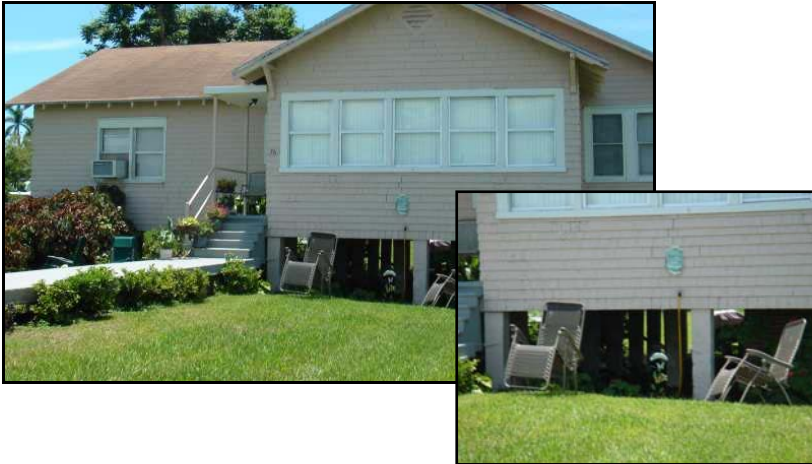
Figure 4 shows a house in the Glades Communities, with an exposed foundation due to the impacts of land subsidence. The second overlay picture shows a close up of the foundation of the house. Source: CSA, 2006.
