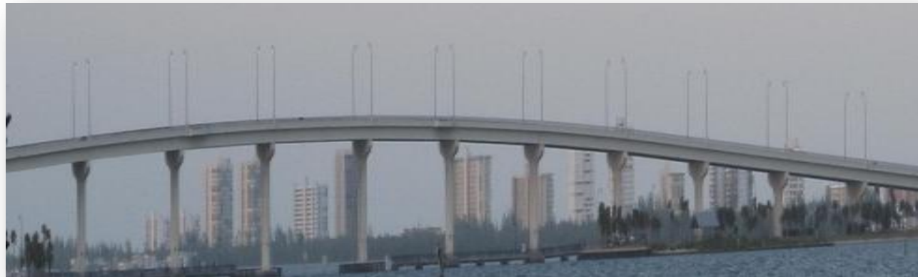
Photo (left): High Span Martin County Intracoastal Waterway Bridge, Helene Wetherington, Calvin, Giordano and Associates, Inc. (2010).
