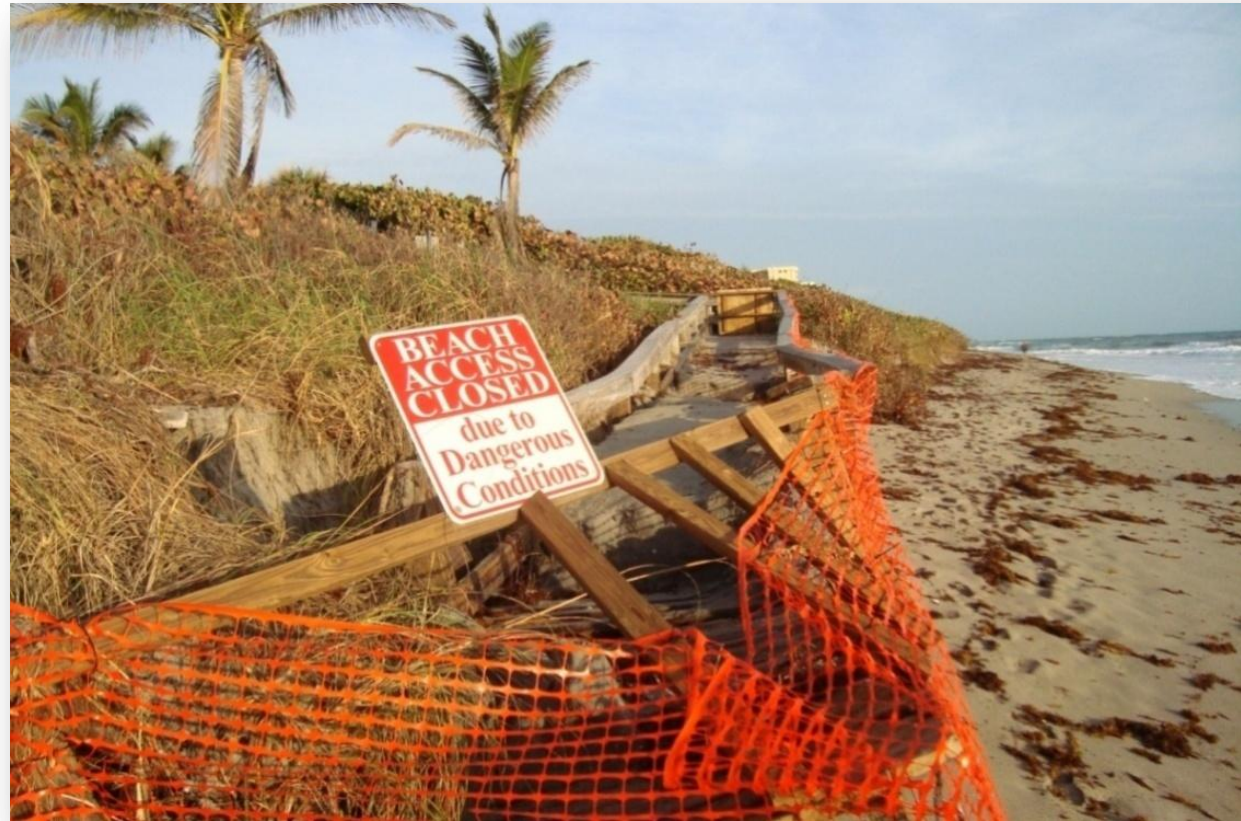
Photo (above): Jupiter beach access damaged by erosion, Nathan Schaeffer, Calvin, Giordano and Associates, Inc. (2011).
