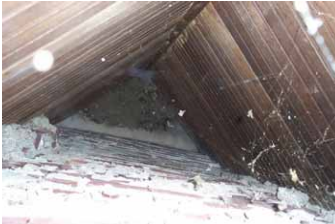
103: Void behind chimney
