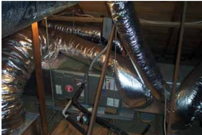
99: Attic HVAC Unit
