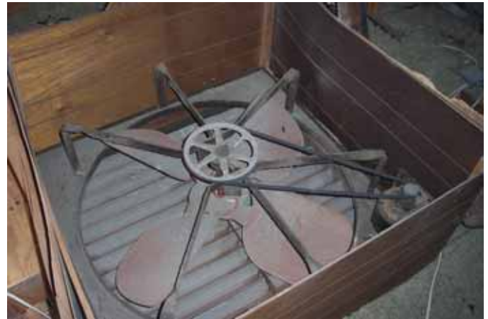
102: "Whole House" Fan in Attic
