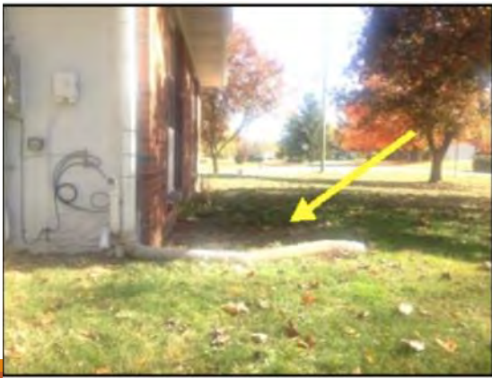
Slope towards foundation
