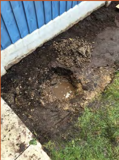
High water table near house
