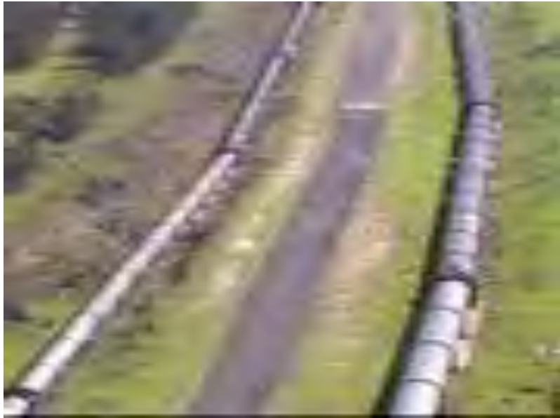
High Pressure Pipelines
