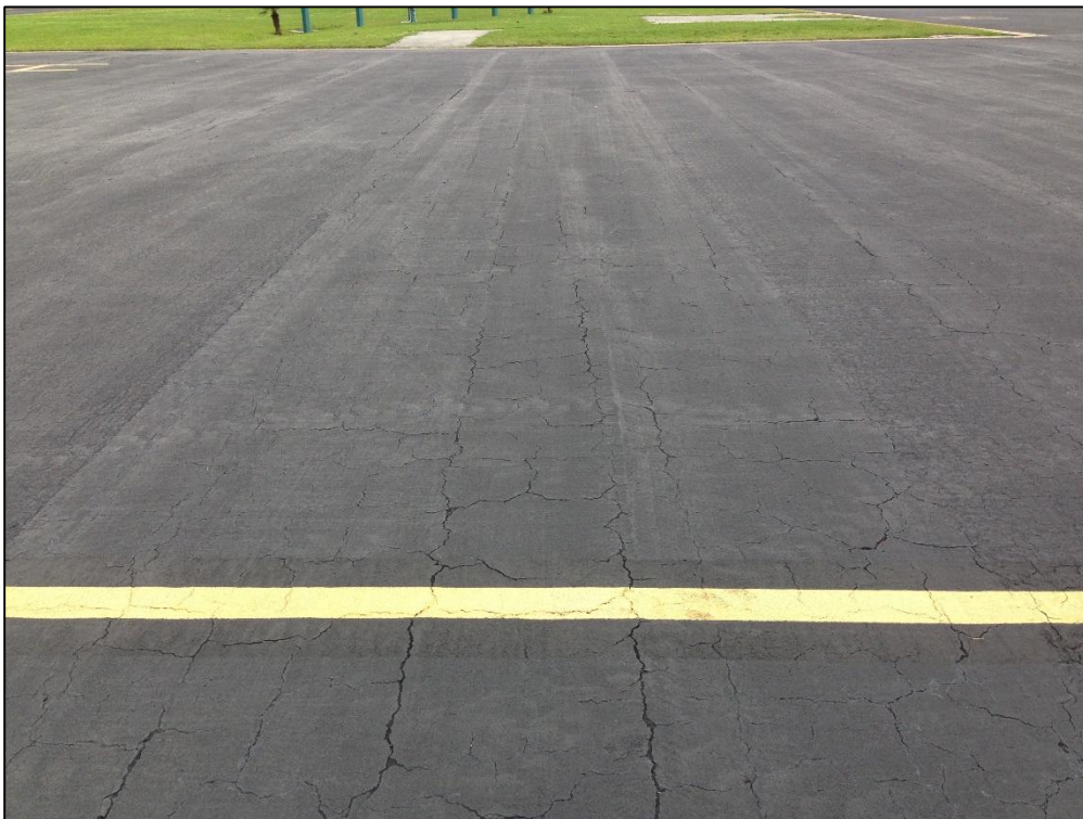
Apron North, Section 4145, Sample Unit 416 – Medium Severity (43) Block Cracking, Low Severity (57) Weathering, Medium Severity (57) Weathering
