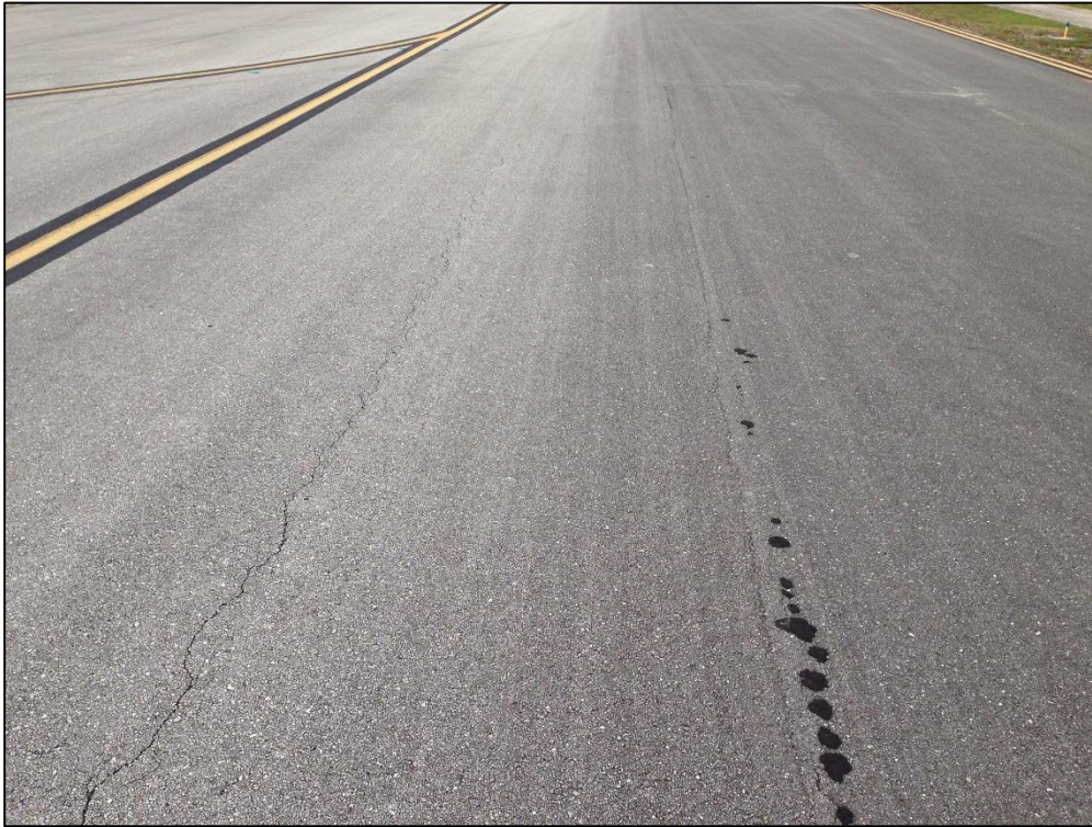
Taxiway Alpha, Section 125, Sample Unit 116 – (42) Bleeding, Low Severity (48) Longitudinal and Transverse Cracking, Low Severity (56) Swelling, Low Severity (57) Weathering
