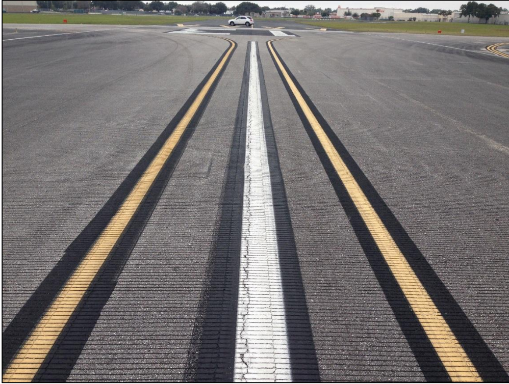
Runway 13-31, Section 6205, Sample Unit 195 – Low Severity (48) Longitudinal and Transverse Cracking, Low Severity (57) Weathering
