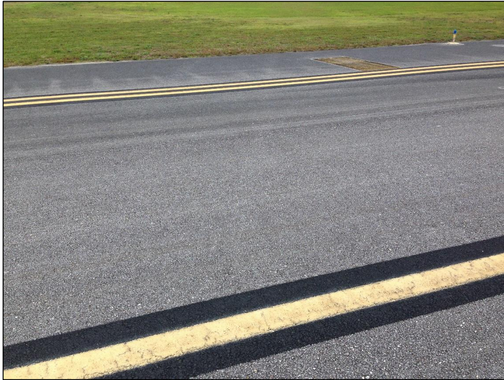
Taxiway E5, Section 560, Sample Unit 101 – Low Severity (52) Raveling, Low Severity (57) Weathering
