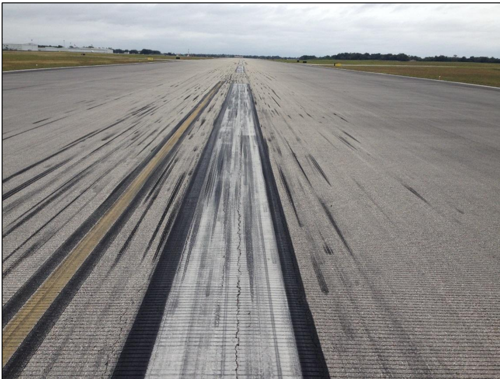
Runway 7-25, Section 6105, Sample Unit 342 – Low Severity (48) Longitudinal and Transverse Cracking, Low Severity (57) Weathering
