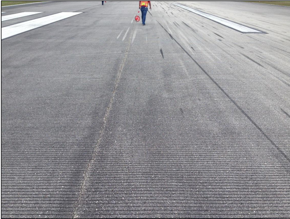
Runway 7-25, Section 6105, Sample Unit 409 – Low Severity (48) Longitudinal and Transverse Cracking, Low Severity (56) Swelling, Low Severity (57) Weathering
