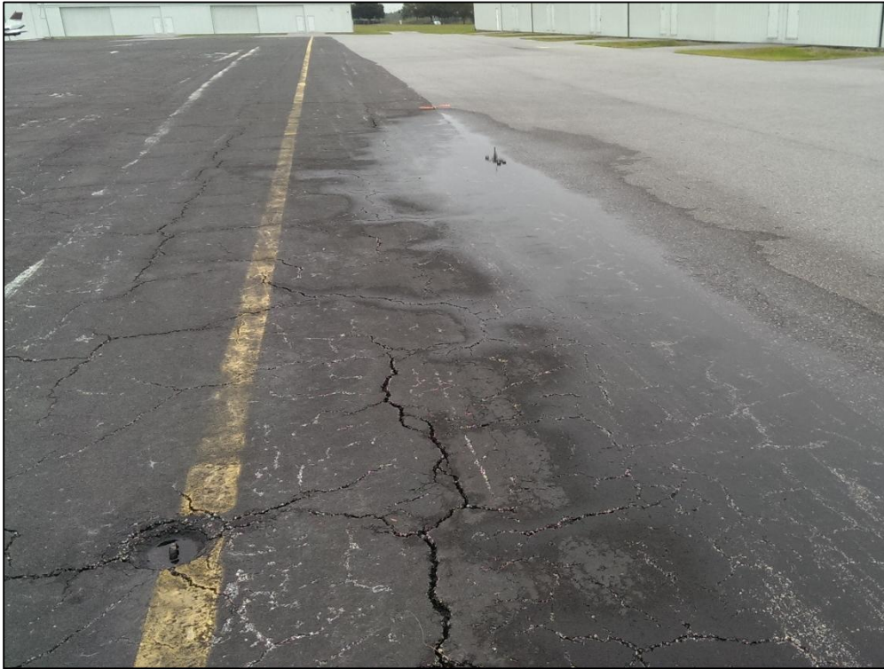
Apron Northeast, Section 4305, Sample Unit 350 – Low Severity (43) Block Cracking, Low Severity (53) Rutting, Low Severity (57) Weathering
