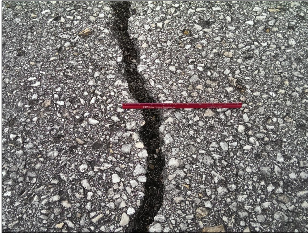
Taxiway E6, Section 805, Sample Unit 801 – High Severity (48) Longitudinal and Transverse Cracking, Low Severity (52) Raveling
