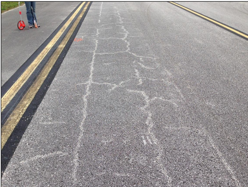
Taxiway Golf, Section 705, Sample Unit 701 – Low Severity (43) Block Cracking, Low Severity (52) Raveling, Low Severity (56) Swelling
