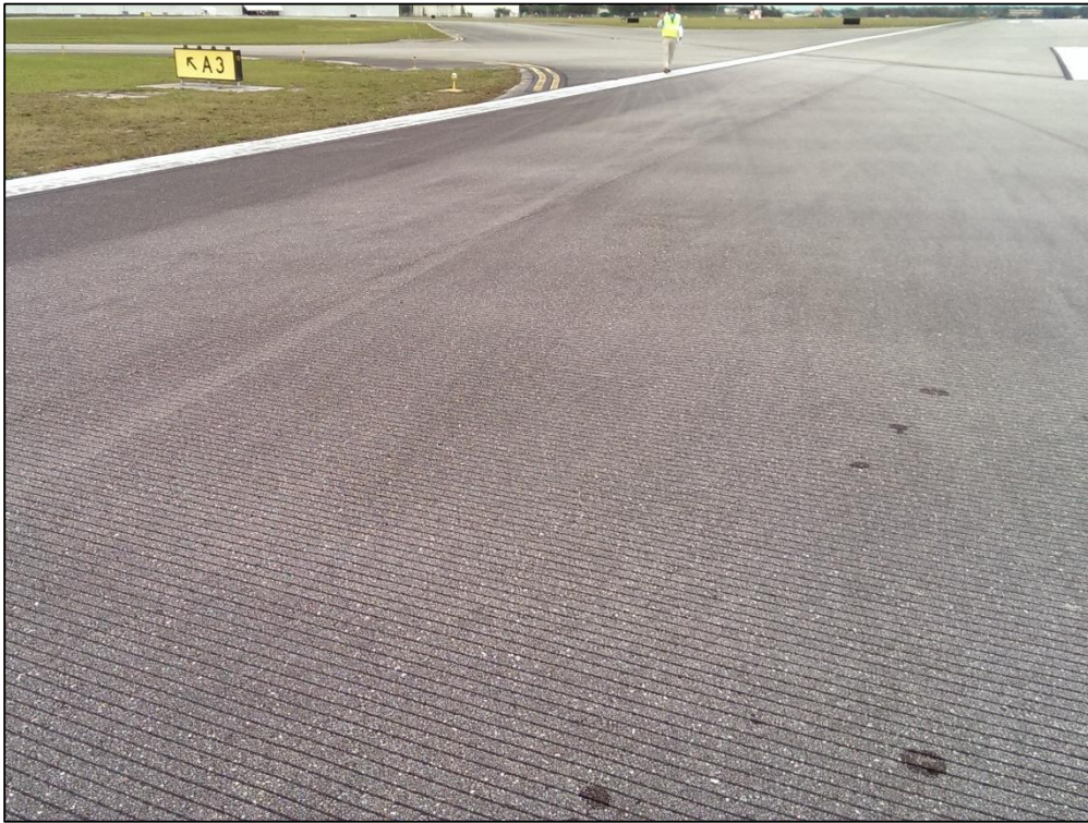
Runway 7-25, Section 6110, Sample Unit 176 – Low Severity (48) Longitudinal and Transverse Cracking, Low Severity (57) Weathering
