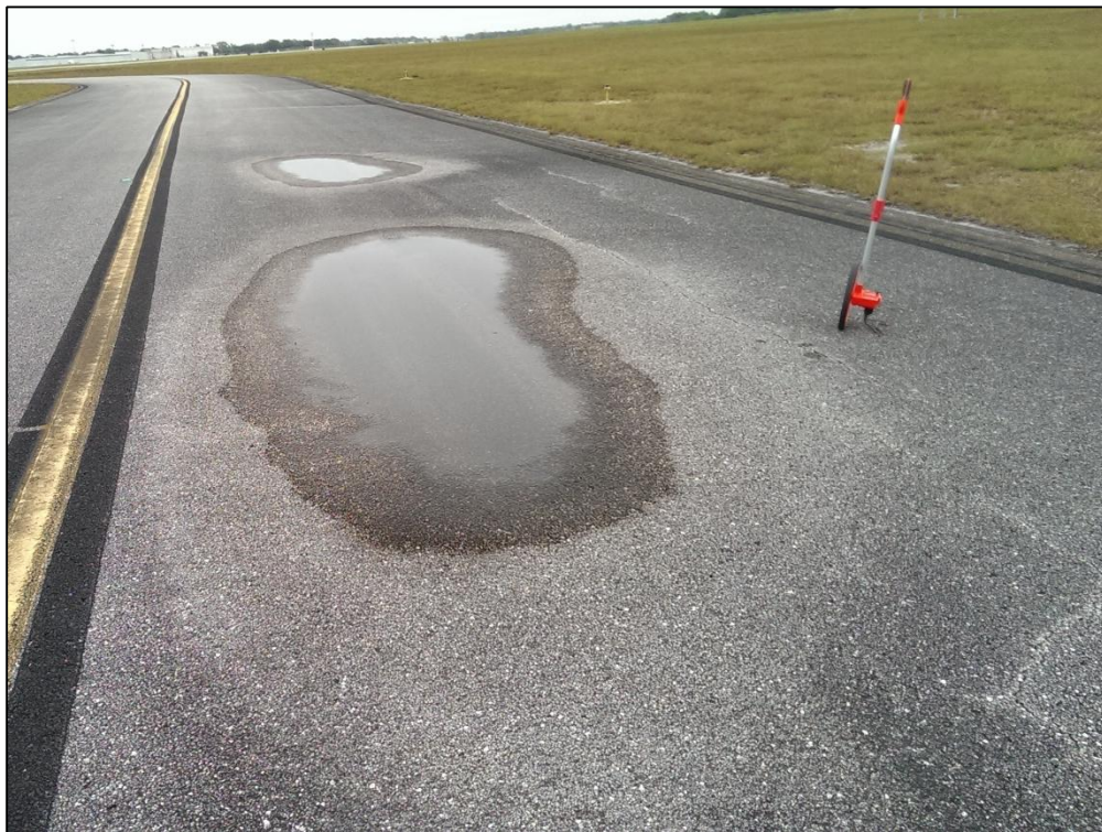
Taxiway E3, Section 420, Sample Unit 405 – Medium Severity (45) Depression, Low Severity (48) Longitudinal and Transverse Cracking, Low Severity (52) Raveling, Low Severity (57) Weathering
