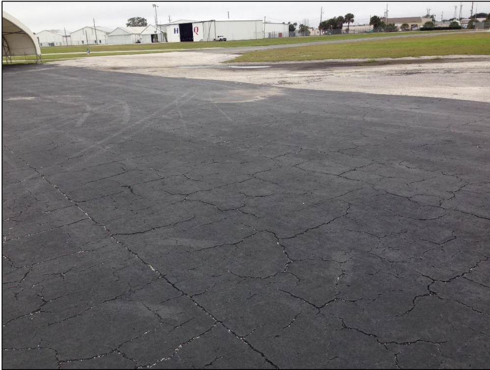
Apron North, Section 4158, Sample Unit 651 – High Severity (43) Block Cracking, Medium Severity (52) Raveling
