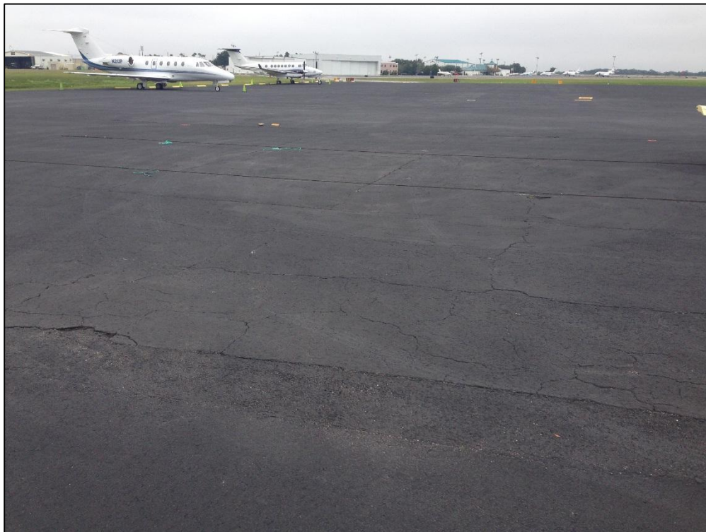
Apron West, Section 4660, Sample Unit 507 – Medium Severity (43) Block Cracking, Low Severity (52) Raveling
