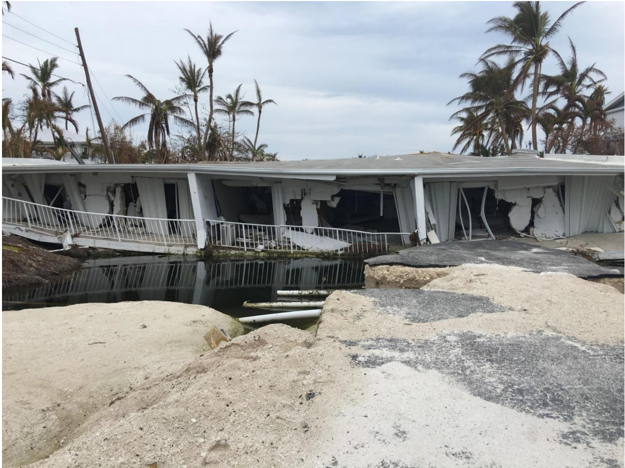
12-Unit Townhouse on Lower Matecumbe damaged by storm surge of Hurricane Irma (Source: Village of Islamorada).
