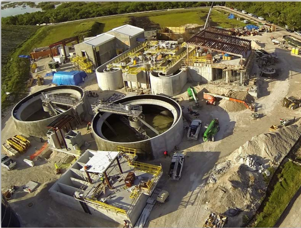
Cudjoe Wastewater Treatment Plant August 2014 (Source: Monroe County)
